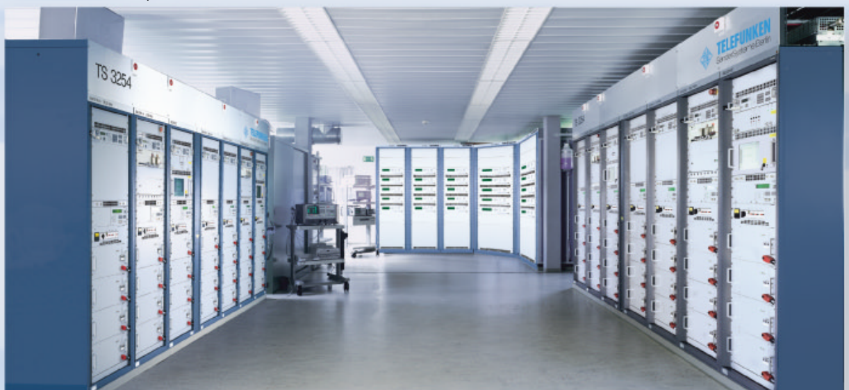
VHF/FM transmitter plant
