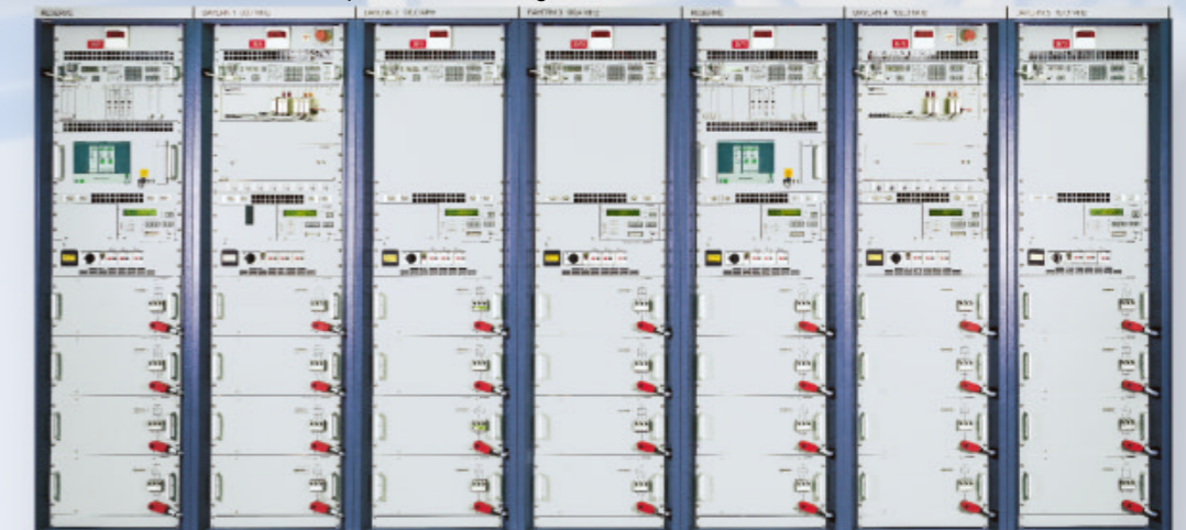
10 kW VHF/FM transmitter plant (n+1 configuration)
